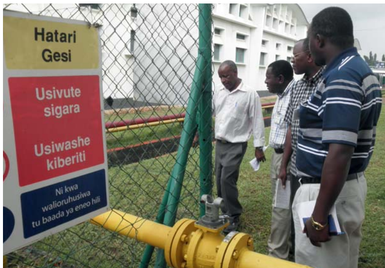
Natural gas infrastructure at Tanzania Cigarette Company Limited in Dar es Salaam. A Cost of Service Study (COSS) to establish costs involved in generation of electricity from gas after completion of a bigger gas pipeline will be instituted.
