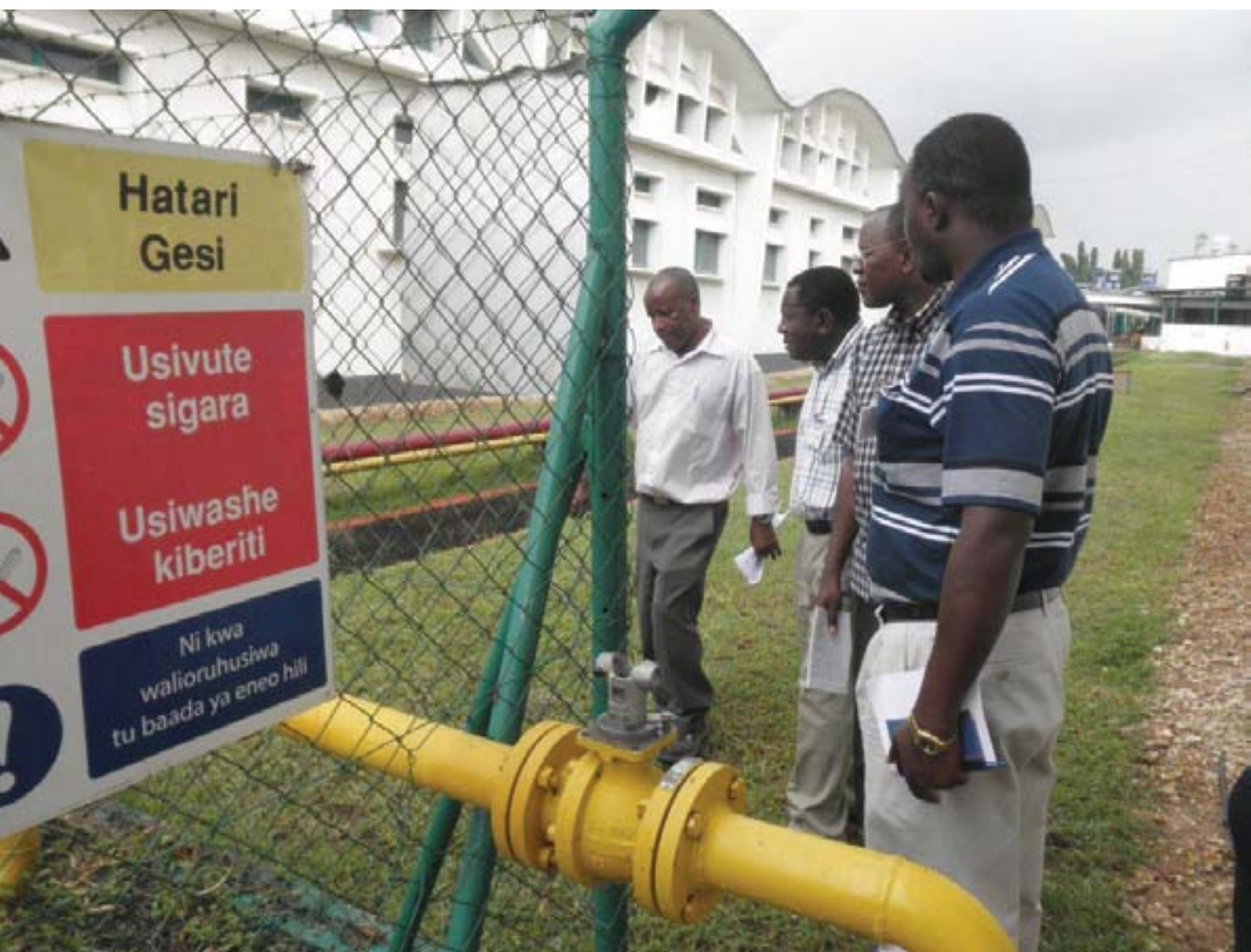
EWURA board member, Mr Nicholaus Mwanji (2nd from left), EWURA's Director of Natural Gas Eng. Charles Omujuni (2nd right), EWURA's Manager for Gas Distribution Eng. Thobias Rwelamila (right), inspect Natural Gas distribution infrastructure at the Tanzania Cigarette Company Limited, in Dar es Salaam, as their host (far left) looks on.
