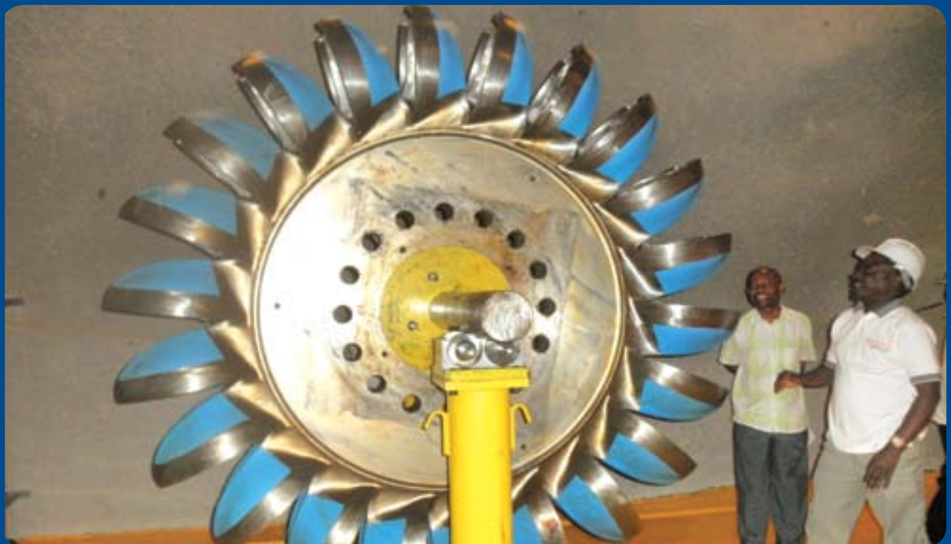
EWURA's Director for Economic Regulation, Mr. Felix Ngamlagosi (capped), observes a power generation turbine at Kihansi Hydro Power Plant on 14th September, 2012, as the plant Manager, Eng. Pakaya Mtamakaya looks on.
