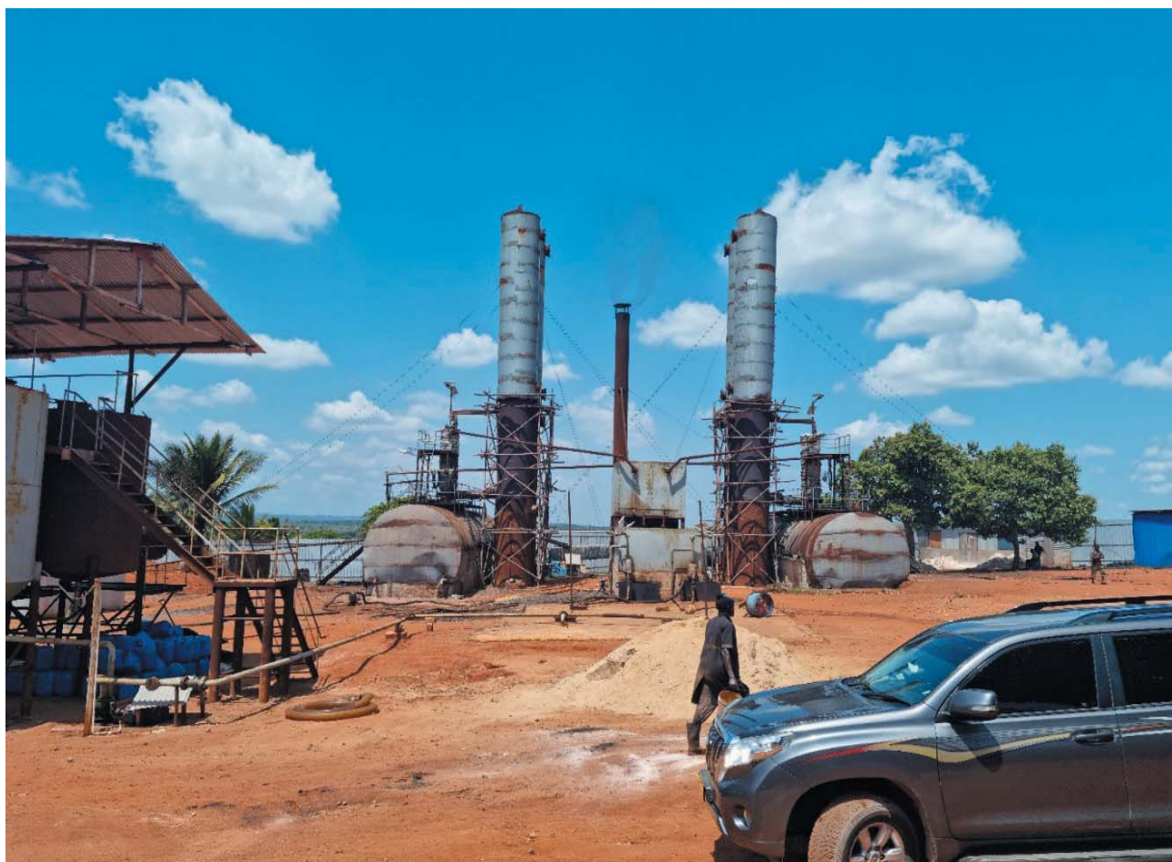
Figure 32: A view of M/S Guoyang Biotech Company Limited's waste oils recycling plant
