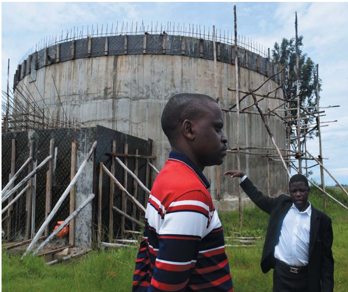
In water tariff setting, EWURA takes into consideration the cost of production and distribution of services, reconnection fee; and investment costs in the infrastructure, such as this water tank which is under construction by Bukoba Water Utility.
