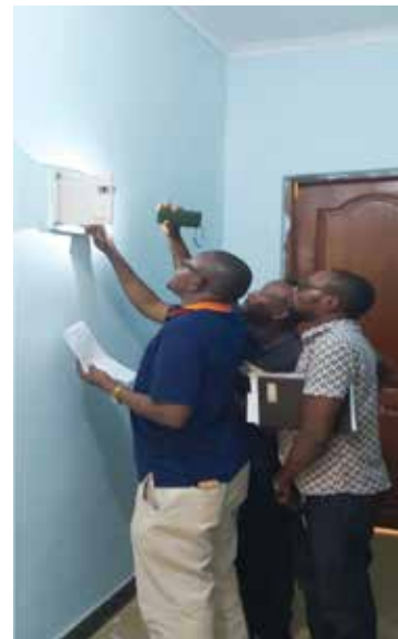
The Electricity official from EWURA, Eng. Evarist Simon (left) inspecting a main switchboard and contexts of the service line application form during visit to one of the TANESCO customer's house located at Mitundurini Street in Singida region. Others are two licensees; Mr. Omary Hamisi Mtaturu and Haruna Jumannne (right) who are EWURA's class C electrical installation licensees.
