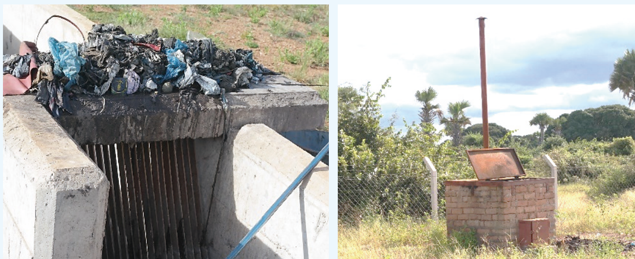
Figure 4- 8 : Solid waste collected at bar screen (left) and a typical incinerator (burning chamber) (right)-Kahama
